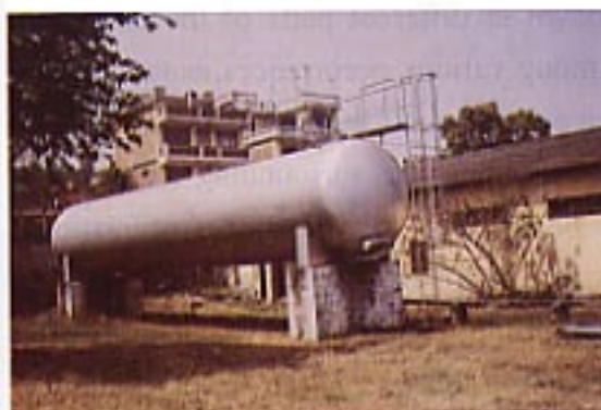
Model Gas Storage Tank, Kathmandu
