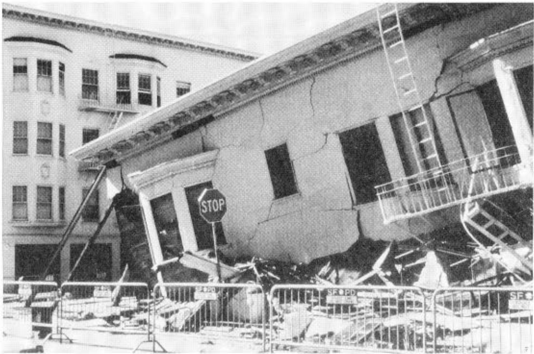
Fig. 9. Photograph from the NGDC slide set collection depicting damage from the Loma Prieta earthquake of October, 1989
