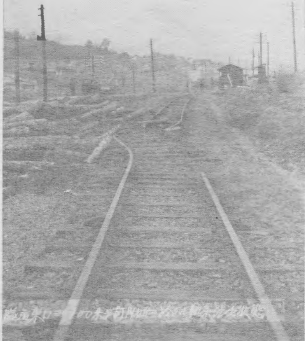
Fig. 2. The fissure limiting the eastern margin of the sliding area and the curved rails at the point 100 meters east of the east entrance of the Kamenose tunnel. (Early in Feb.)
