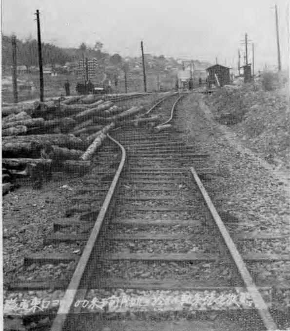
Fig. 2. The fissure limiting the eastern margin of the sliding area and the curved rails at the point 100 meters east of the east entrance of the Kamenose tunnel. (Early in Feb.)
