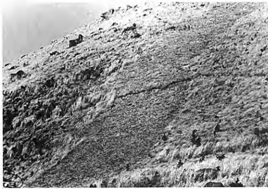
2. 浅間山南西斜面に生じた亀裂 ↑ Detail of the same point as Plate 12-1.
