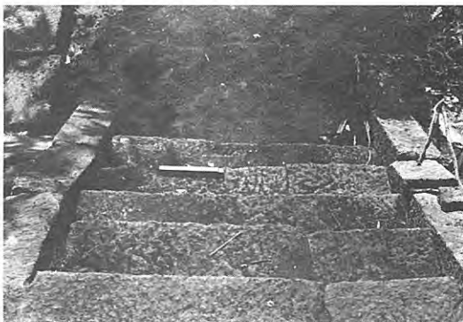
5. 小さな右横ずれ変位を示す愛宕神社の石段 Slightly right-lateral displacement of staircase by faulting at Loc. 23.
