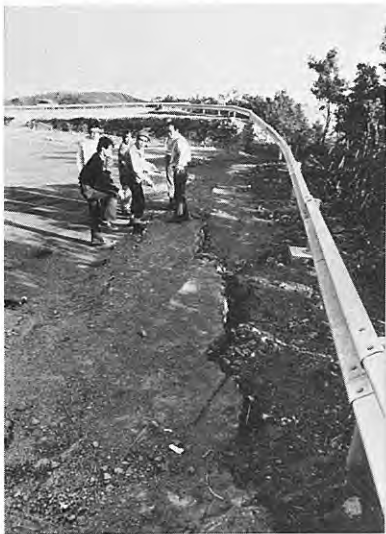
3. Cracks in a parking place at loc. 70.
