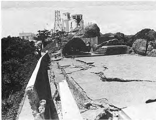
1. Damaged road and masonry house at Irozaki (loc. 64).
