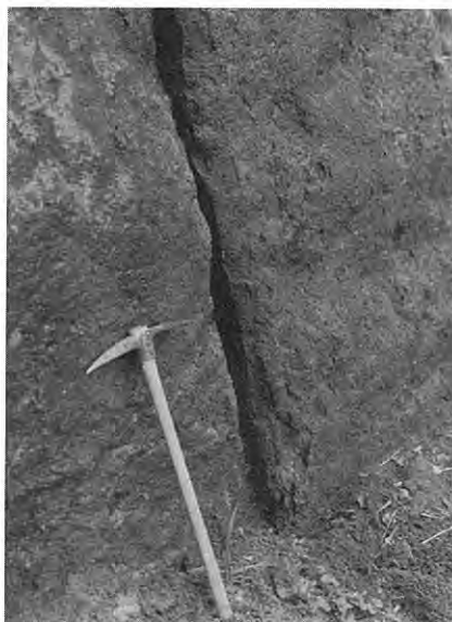
2. Subsidiary earthquake fault exposed in a cutting wall at loc. N-1 (Irozaki-north fault).
