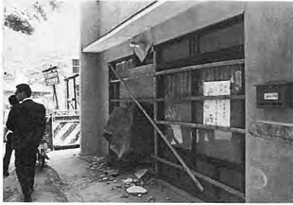
1. Damage to a house by a fallen rock at Shimogamo.
