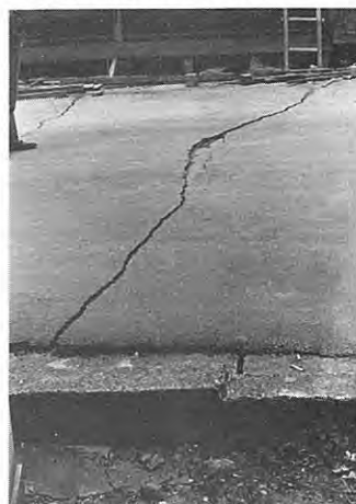
4. Cracked road on the earthquake fault at loc. 4.
