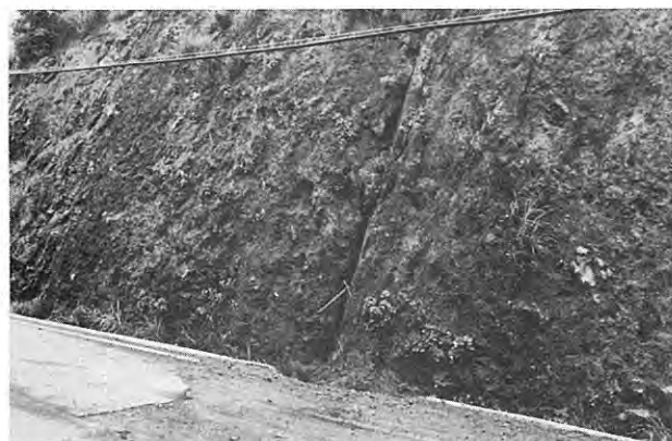
2. Lower part of the same fault as photo. 6-1.
