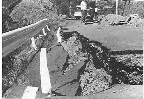
2. Destruction of road by collapse of bed rock (volcanic breccia) at loc. 74.
