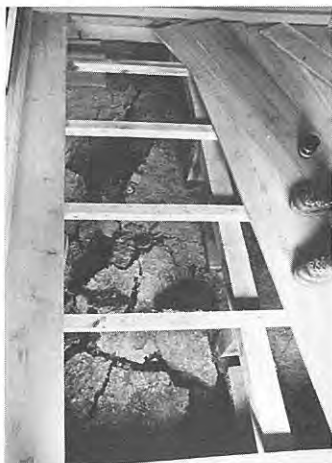
5. Fissures appeared under the floor of a house at loc. 5.
