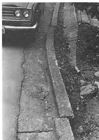
2. Right-laterally displaced road on the earthquake fault at loc. 4.
