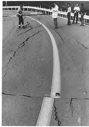
4. Cracks on asphalt road caused by swelling or sliding of embankment at loc. 75.
