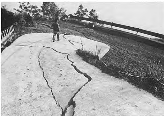
5. Cracks of concrete road on a spur at loc. 71.
