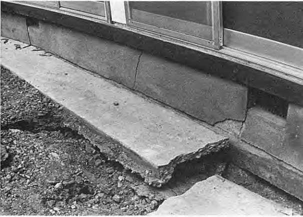
1. Ground crack and damaged foundation of a house at loc. 5.
