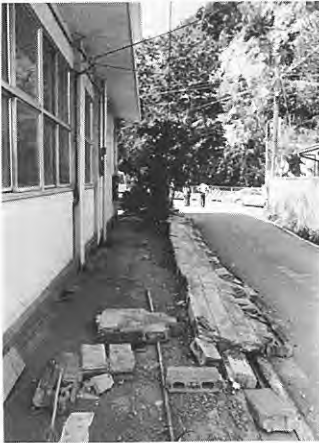
3. Destruction of concrete block masonry fence at Shimogamo.
