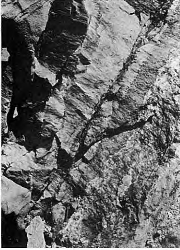
1. Slightly parted bedding fault at loc. 27.
