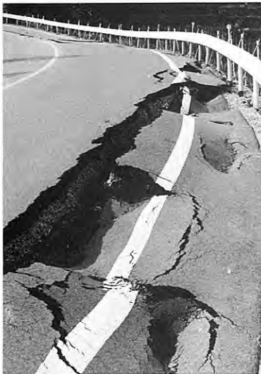
6. Settlement and sliding of road foundation at loc. 75.
