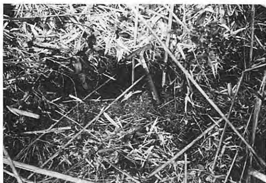
4. Fissure on the slope at loc. 40. South (this)-side down throw is observed.
