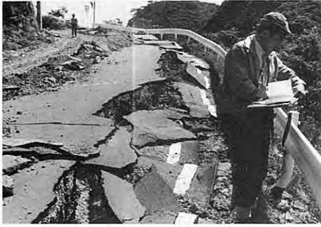
1. Collapse of the road surface at loc. 74.
