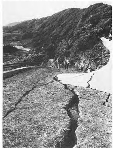
6. Cracks and fissures at loc. 71.
