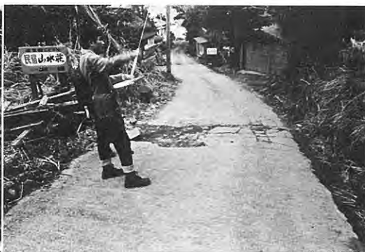
5. Cracked road on the active fault line at loc. 42.
