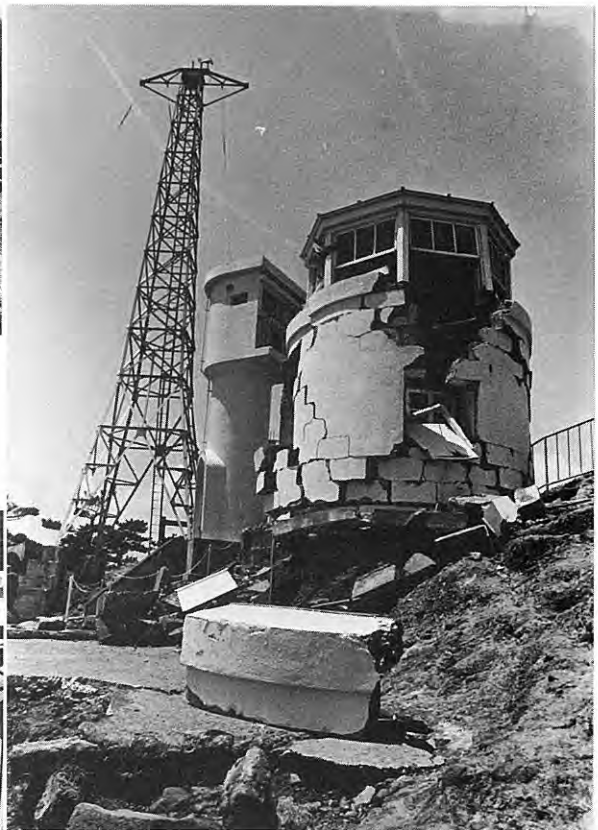
5. Damage to an old masonry watch-tower at Irozaki.
