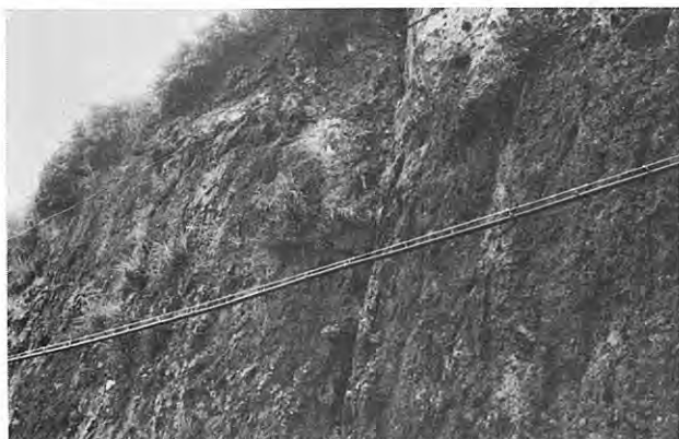
1. Exposed earthquake fault at loc. S-2. Upper part of the northern wall of a cutting.
