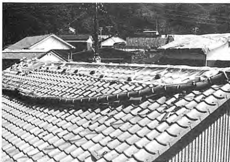
4. Damage to roofs at Mera.
