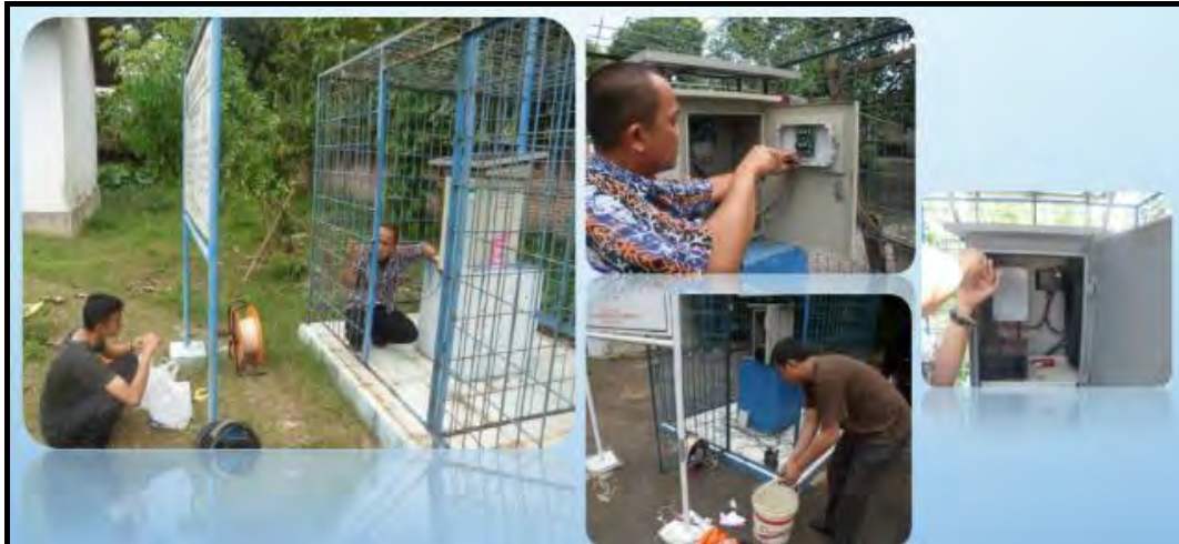
Fig. 10. Maintenance activities of groundwater monitoring wells.
