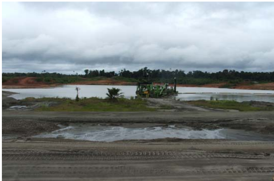
Fig 3 shows mine tailings storage facility of Ok Tedi Mine under construction at Bige in Western Province, PNG
