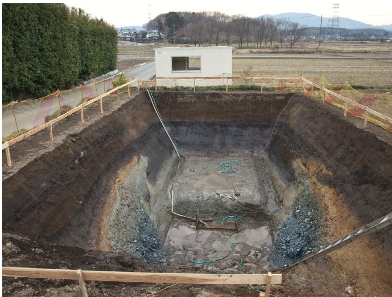
第5図. 掘削が完了したトレンチ. 隆起側(北東側)から低下側(南西側)を望む. Fig. 5. Snapshot of the excavated trench viewed from the uplifted (northeast) side.
