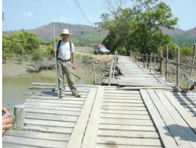
Photo 13. Destruction of bridge to Konnamaing Chaungwa Village by tsunami (narrow flat portion in the right far site of photo).
