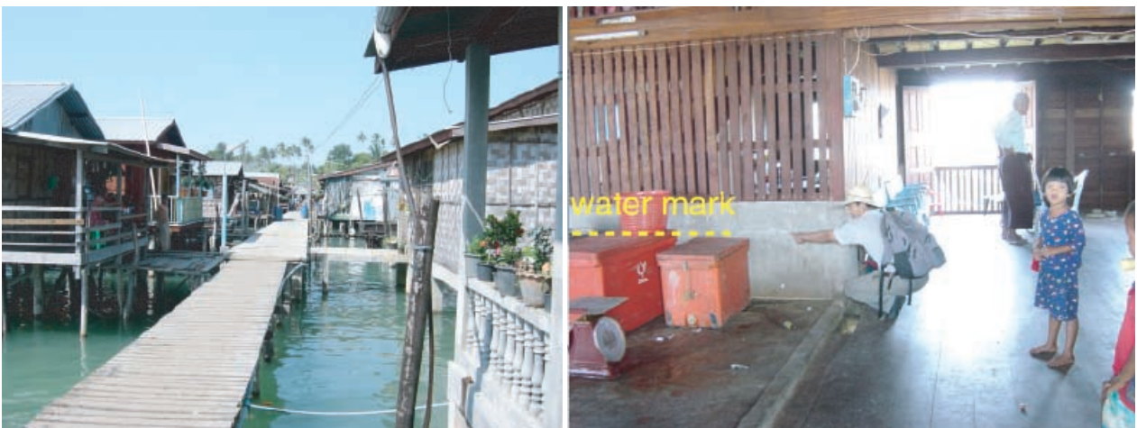
Photo 10. Houses above water (left) and the watermark on the wall of a house (right).
