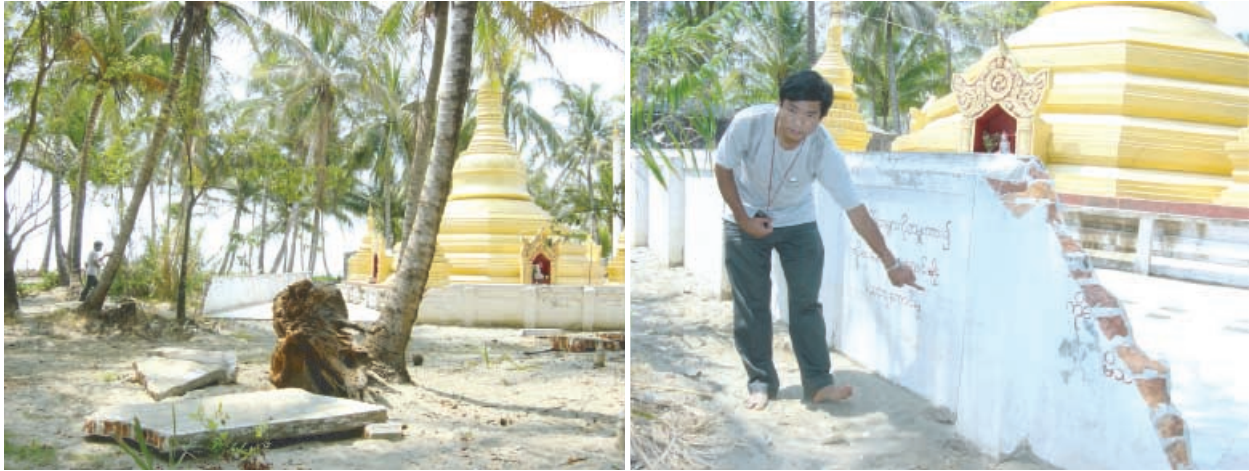
Photo 24. Field survey at Kaing Thaung Island Pagoda. Walls of Pagoda are destructed by Tsunami (left) and Watermark at the wall (right).
