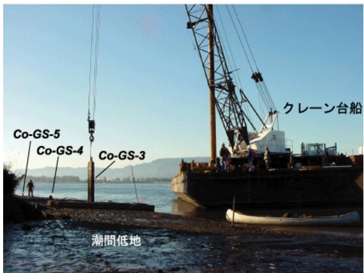
写真3. ジオスライサー引き抜き作業 (Co-GS-3) . Photo 3. Pulling out the sheetpile and shutter plate, which are bolted together at top.
